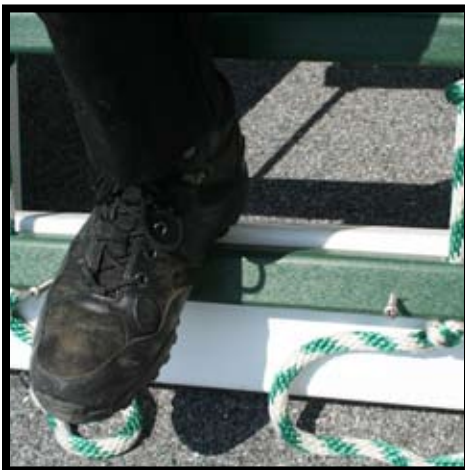
Finish installation by starting two 1/4" x 3" screws, and pushing the base block down with your full weight. Drive screws into ground rail.
